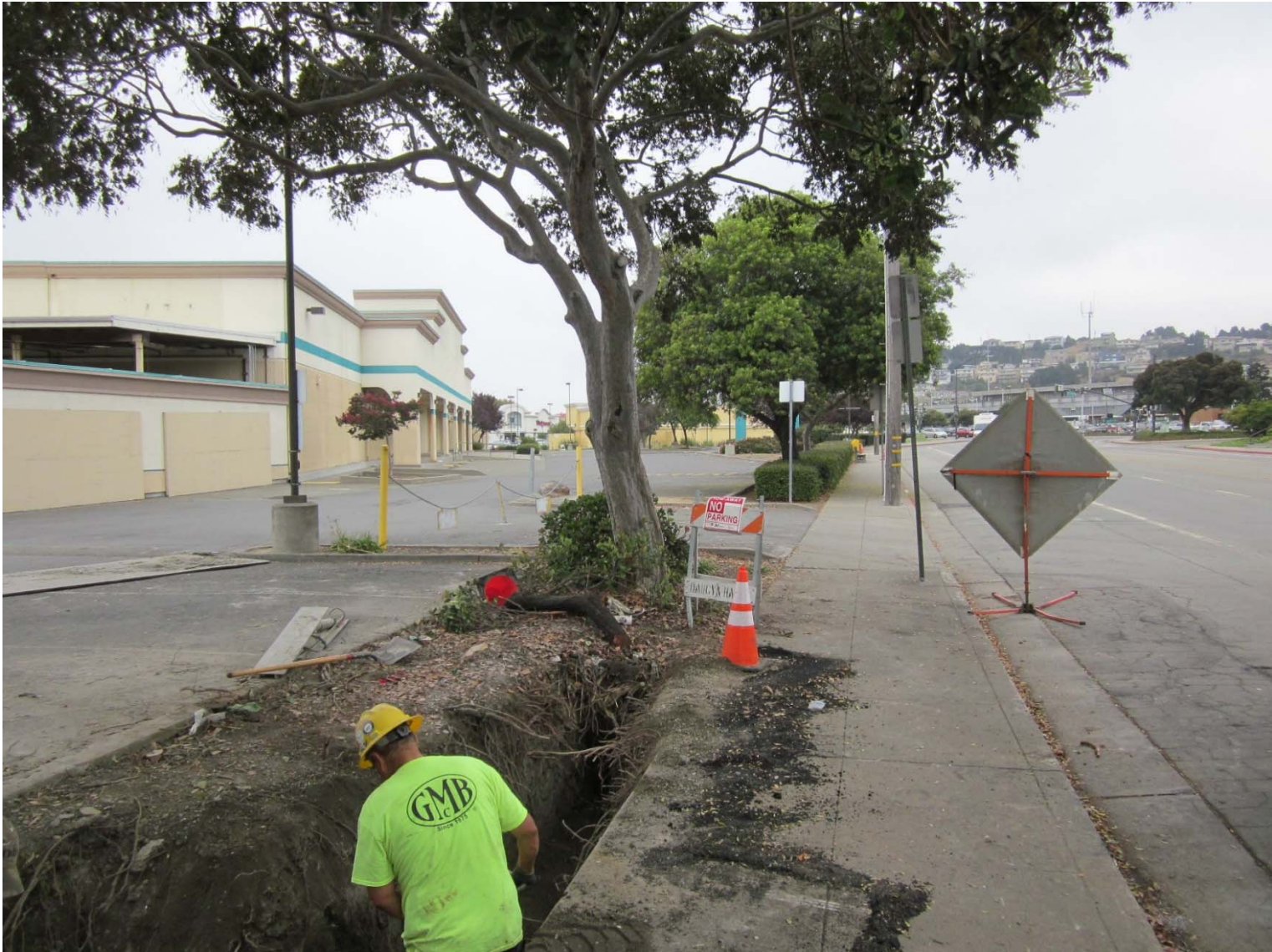
2017 Pipe Burst by District Contractor
